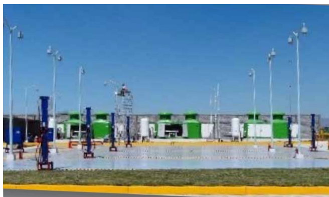
Pressure reduction and truck refueling station Mexico
